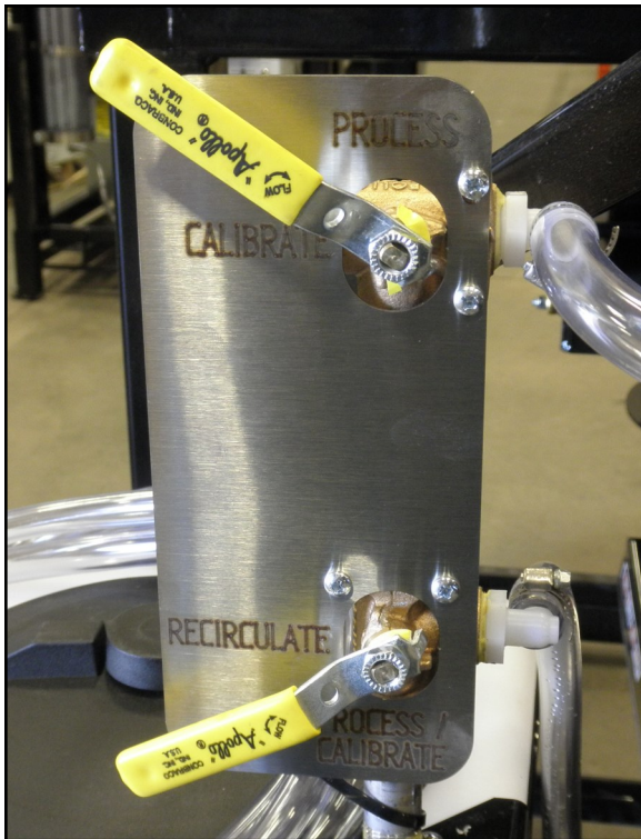
Left Tank Source Valve
