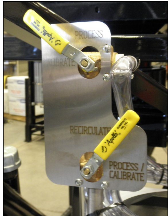
Right Tank Source Valve
