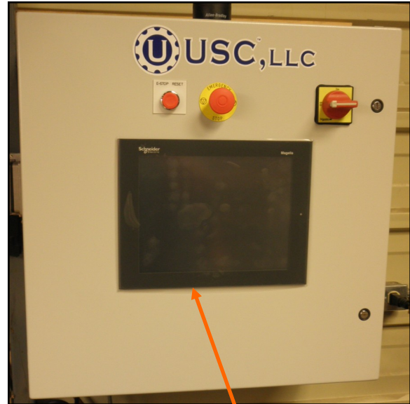
HMI screen on LPX Automated Control Panel
