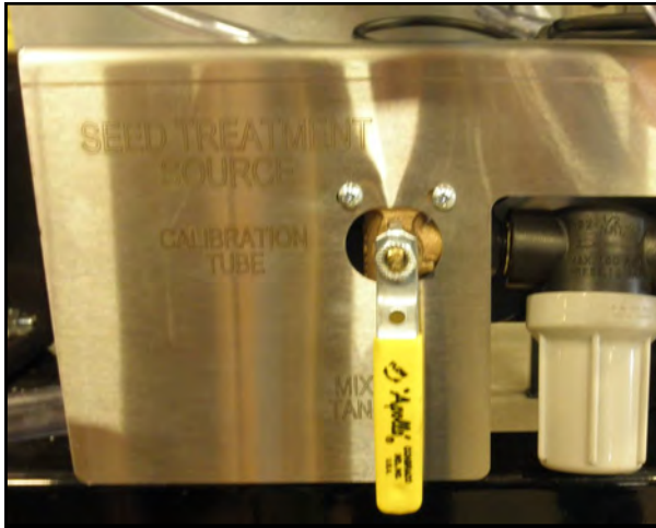
Pump #1 Drawing from bottom of Mix Tank
