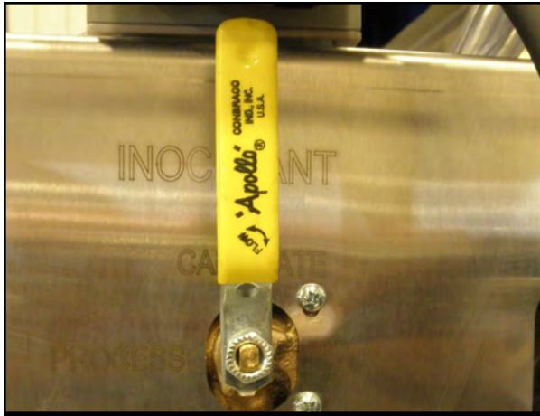
Pump #2 Pumping Liquid to Calibration Valve
