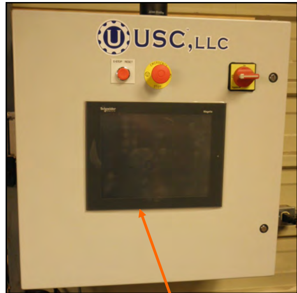
HMI screen on LPX Automated Control Panel
