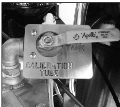
Pump #1 pumping liquid into the top of the mix tank when Seed Treatment Valve is in Calibrate.
