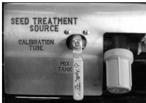
Pump #1 Drawing from bottom of Mix Tank
