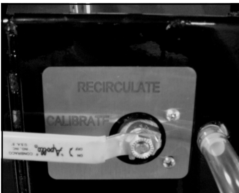
Directs liquid to the hose to the right of the valve to check calibration
