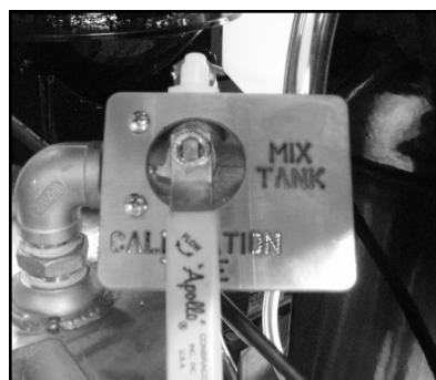
Pump #1 pumping liquid into the top of the calibration tube when Seed Treatment Valve is in Calibrate.
